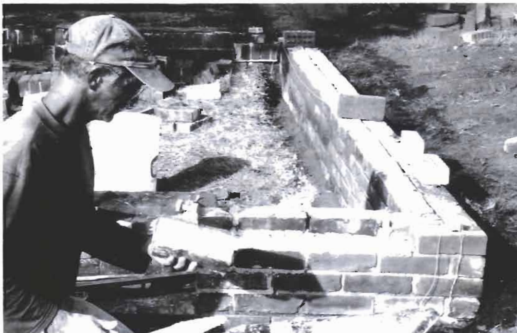
Bo Patterson hard at work repairing a brick wall in Linwood Cemetery.
